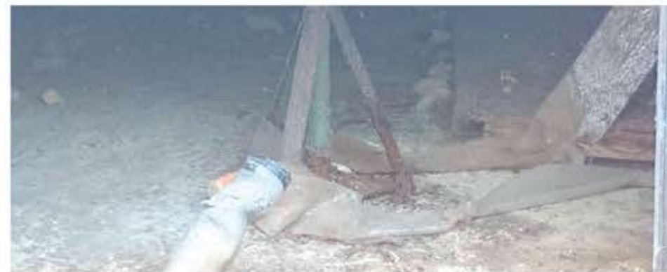
Above: Rusty supports and chassis underneath Steve Wall's park home. It's clear to see that Park Home Chassis Services needed to act promptly here
